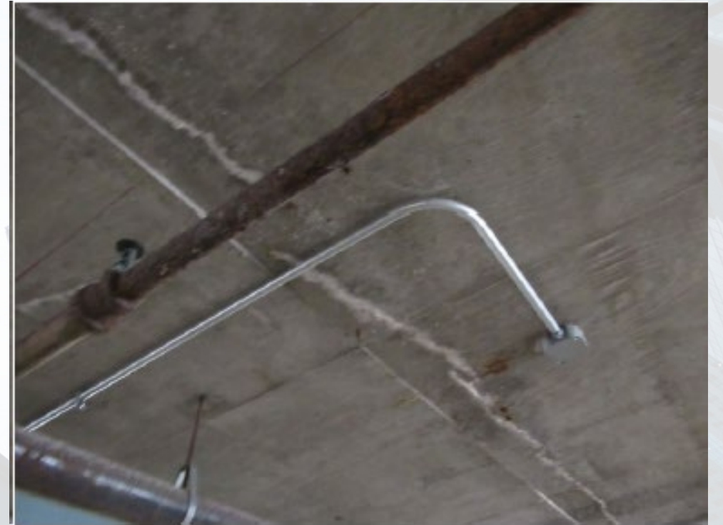
Evidence of water infiltration beneath elevated garage floor
